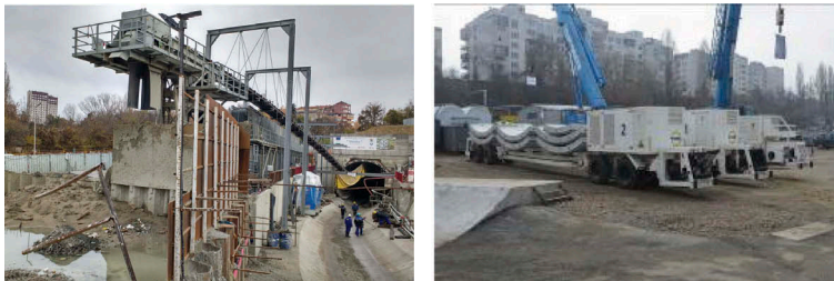
Figure 6. Main tunnel conveyor on launching site, and MSVs used in the Project.
