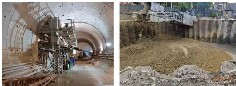
Figure 8. Belt conveyor exiting from the main tunnel and ancillary inclined belt conveyor mucking out.
